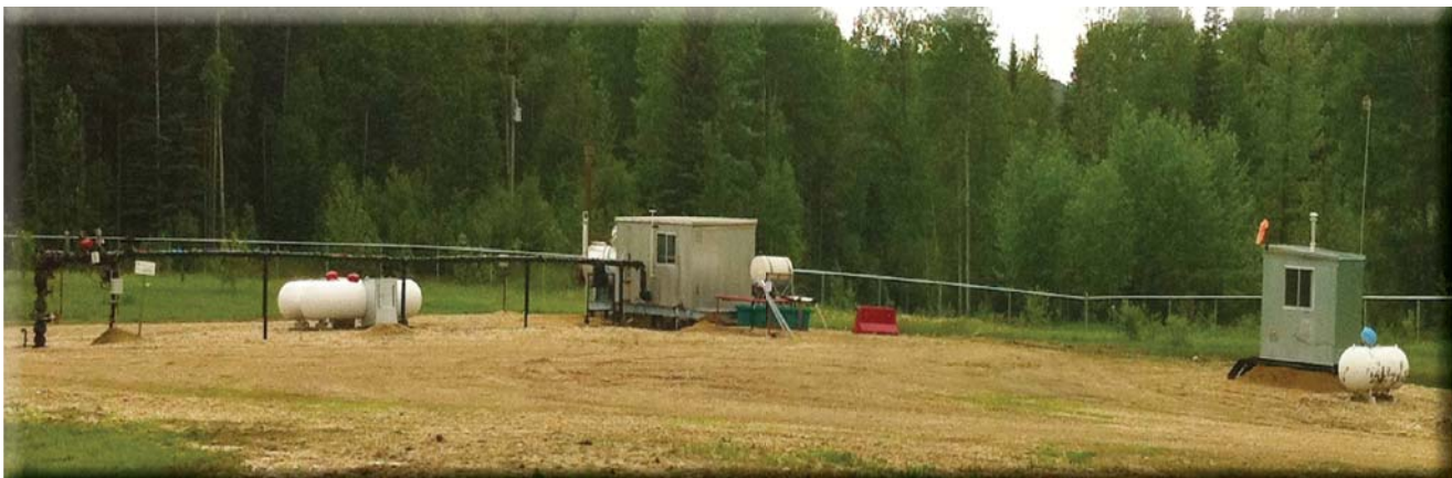
Natural gas facility
